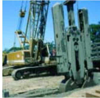
▲ A slurry wall panel excavator is used to dig the foundations for the 69 panels in the memorial.
