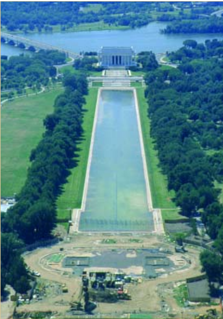
▲ Crews begin work on the World War II Memorial in Washington, D.C.
