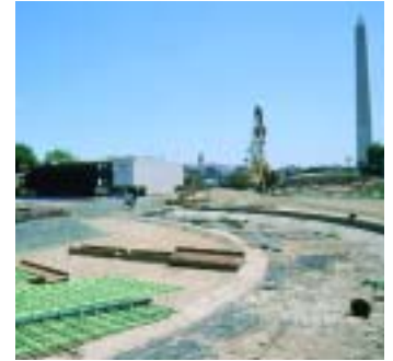
▲ Steel beams and rebar cages are prepared for use in the construction of the memorial's slurry wall.
